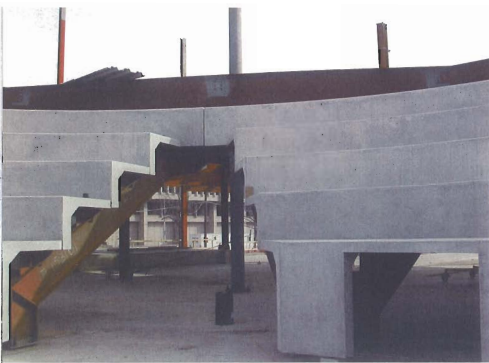
Embedded plates at the tread and riser were welded to steel bearings on sloping steel girders.
